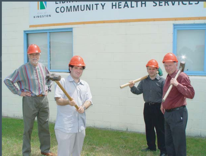
Left to Right: Cr. Arthur Athanasopolous (second left and Peter Spyker CBCHS Board of Management President (far right), with two members of the City of Kingston Access and Equity Committee, start demolition for the new Clarinda site.
